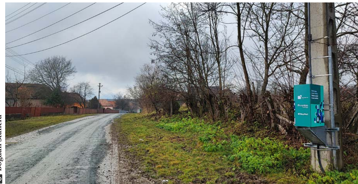
Where the paved road ends, there the broadband starts. For now, the village of Plaiuri has no asphalted road, but the broadband cable just arrived – the box on the right of the image is the local switch.
